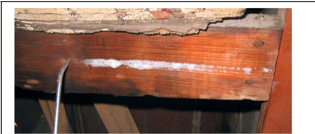
Using the Tornado to deliver treatment along the grain of a beam.
